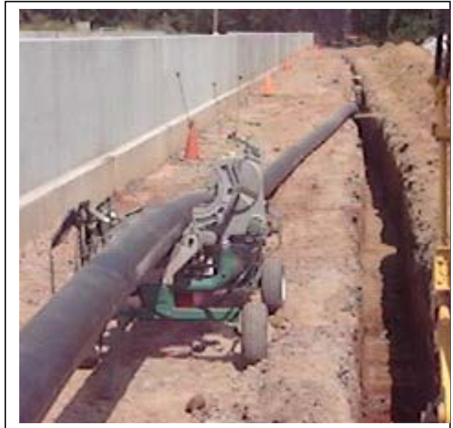
discharge line from the treatment building to a discharge point at an adjacent stream.
